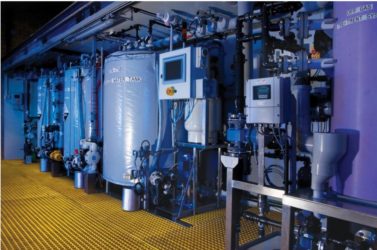
Figure 2 – The PhosEnergy Demonstration Plant
